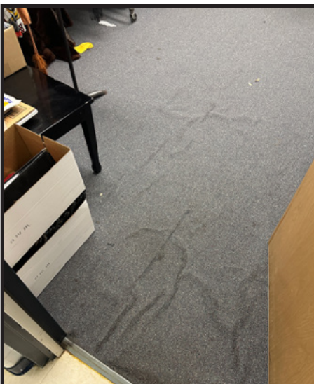
Flooring is dated and damaged, causing safety concerns.
